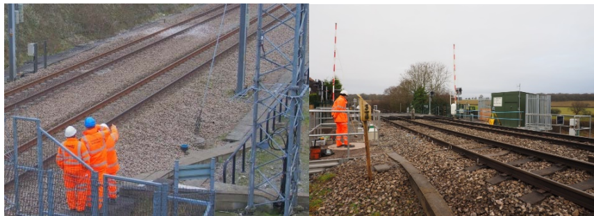
Fig.E1: (a) Rigid and (b) flexible UTX and associated trackbed faults
